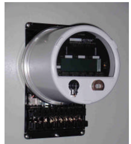
Retrofit VECTRON in Panel
