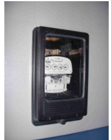
Westinghouse Meter in Panel
