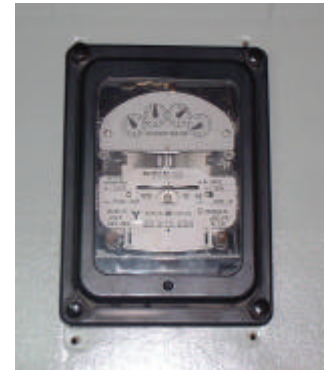
GE Meter in Panel
