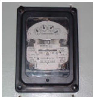
1. GE Meter in Panel
