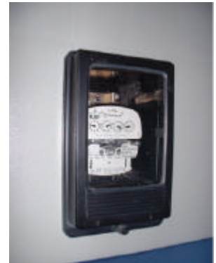
Westinghouse Meter in Panel
