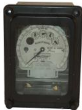
1. GE Meter in Panel
